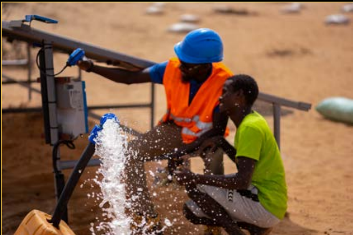
Water flows using solar powered irrigation Senegal
